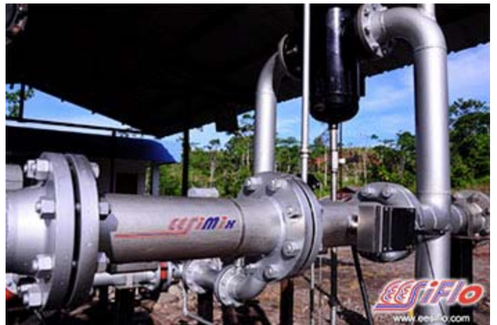
Crude Oil Export Metering Stations
